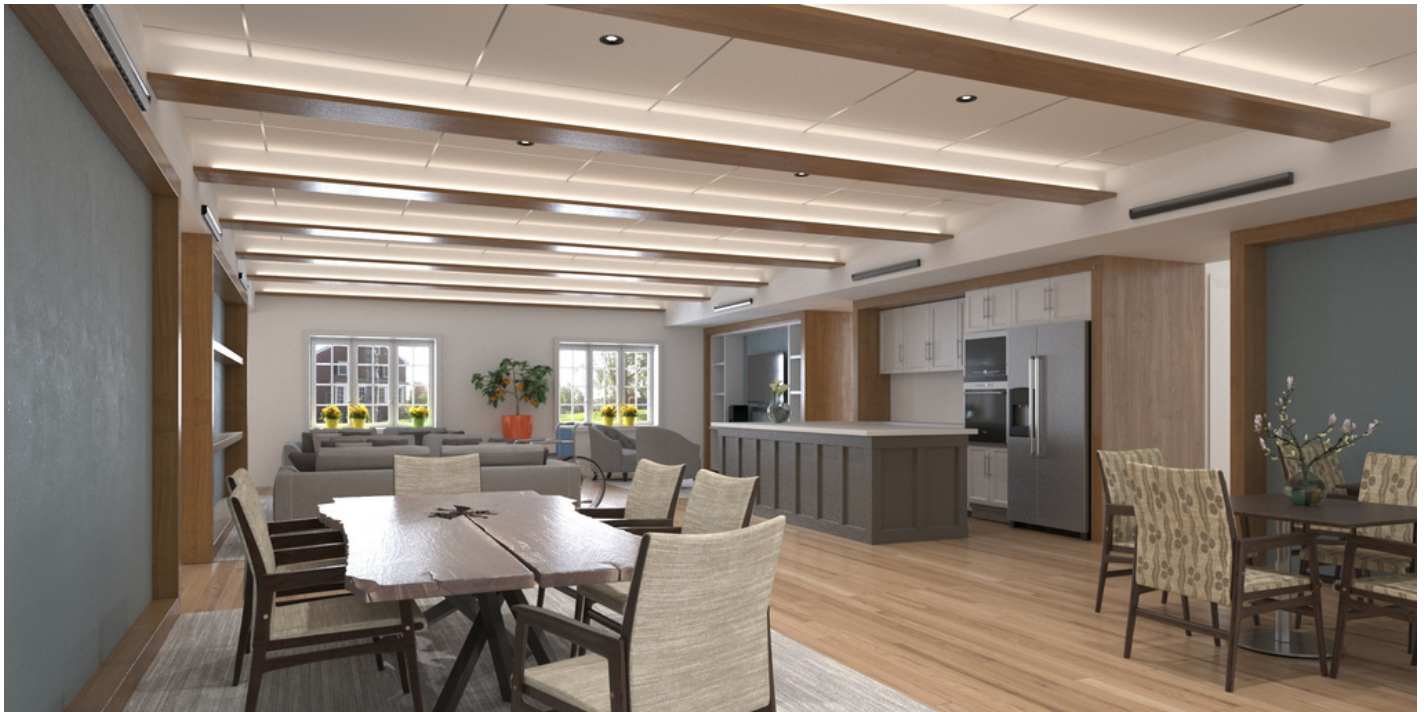
Figure 22: Purifii AER W installed in the common area of a senior living facility.
